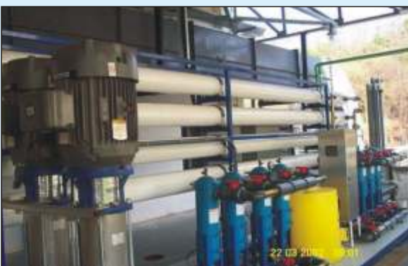
RO SYSTEM FOR WATER TREATMENT AT SCI LTD., MAHAD
